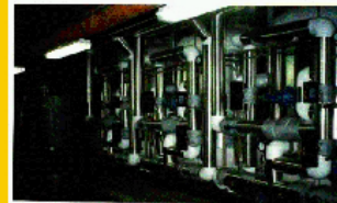
PIPING AND VESSELS
