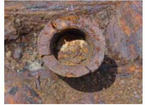
Fractured collar-coupling assembly
