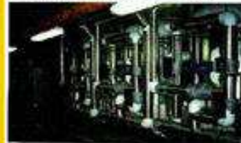
PIPING AND VESSELS
