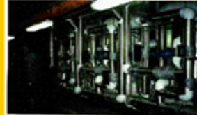
PIPING AND VESSELS
