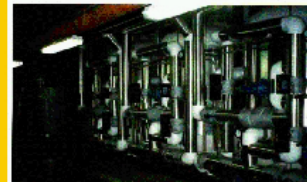
PIPING AND VESSELS
