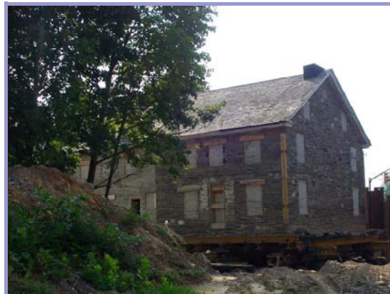
Inching its way to its new home, the 670-ton Tavern gained almost 230 tons during the move, making its total cargo weight just under 900 tons.
